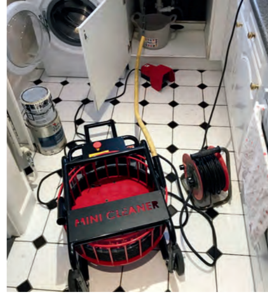
Photo courtesy of MT Drains
